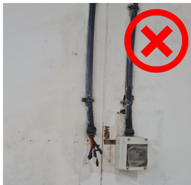
Poor electrical installation
